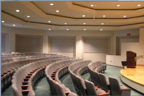
Sound Delete Acoustical Wall Panels on wall to reduce noise reflection
