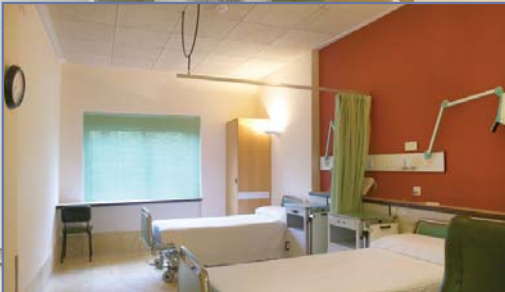
Sound Masking installed above the ceiling tile to mask out noise from outside the room
