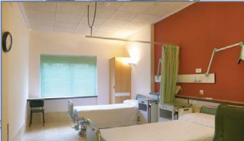
Sound Masking installed above the ceiling tile to mask out noise from outside the room
