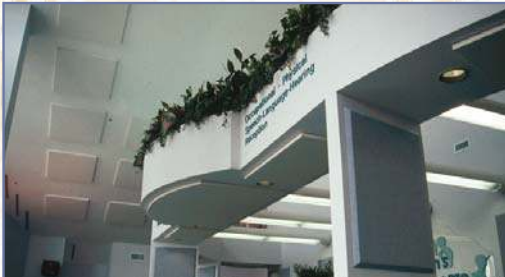
Sound Delete Acoustical Ceiling Panels and Wall Panels to reduce noise reflection of drywall ceiling
